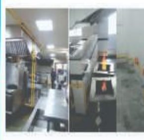
Gas Pipe Line
